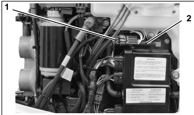
1. CANbus connectors 2. EMM cooling water hose 006744
