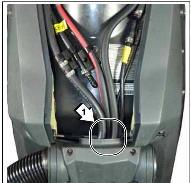
1. Cables NOT pinched 009170
