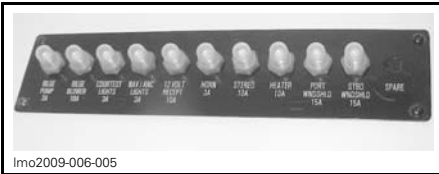
CIRCUIT BREAKER PANEL
