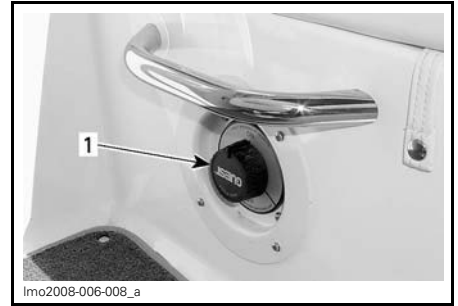
1. Main battery cut-off switch
