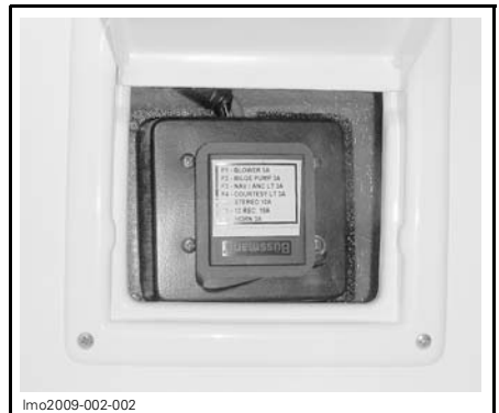
FRONT FUSE BOX
