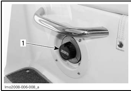
1. Main battery cut-off switch
