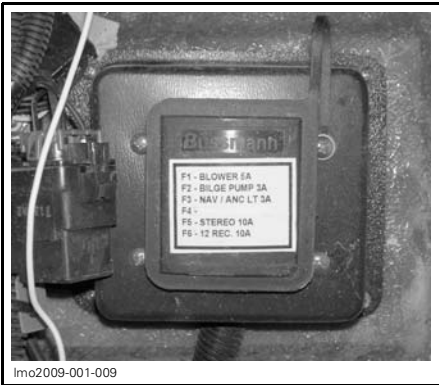
FRONT FUSE BOX
