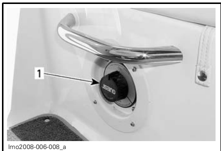
1. Main battery cut-off switch
