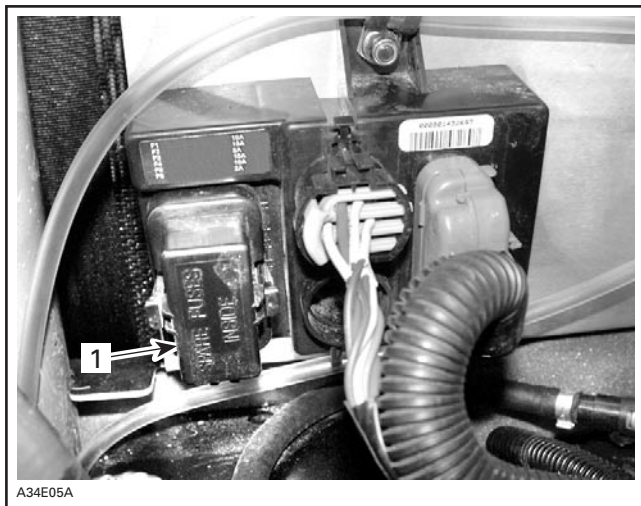
1. Engine fuse box
