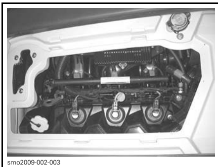
VENTILATION BOX REMOVED
