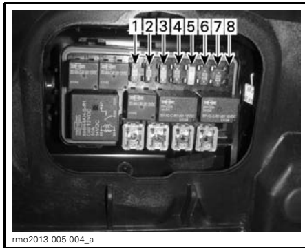
FUSES - RIGHT FUSE BOX
