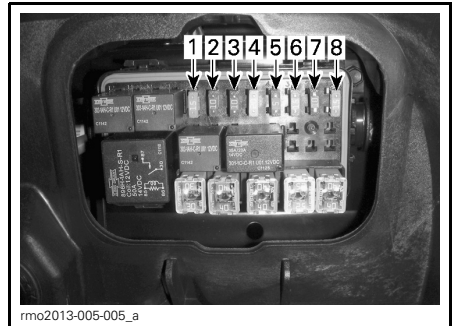
FUSES - LEFT FUSE BOX
