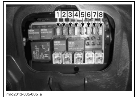
FUSES - LEFT FUSE BOX
