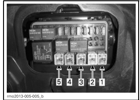
JCASE FUSES - LEFT FUSE BOX
