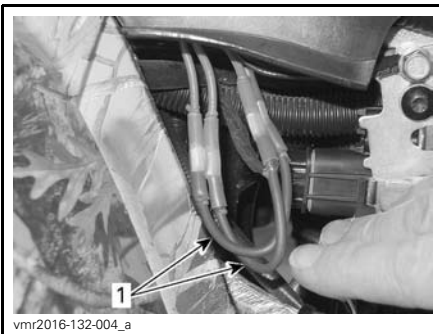
vmr2016-132-004_a 1. Fusible links
