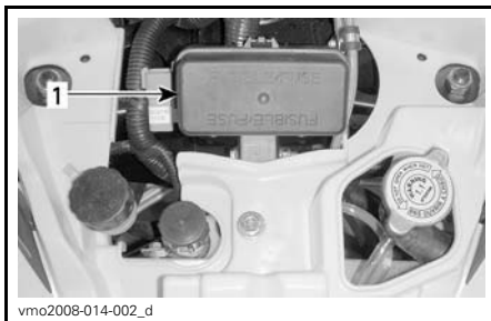
1. Front fuses box
