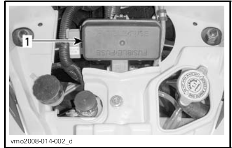
1. Front fuses box
