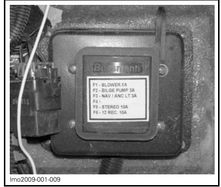
FRONT FUSE BOX
