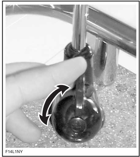
OPEN FAUCET VALVE
