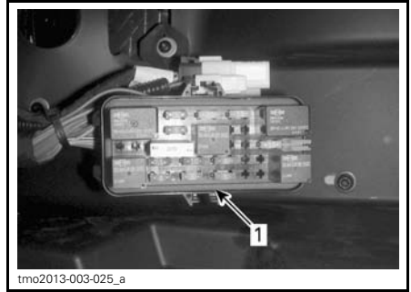
1. Main fuse box
