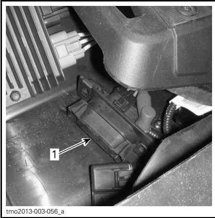
1. Auxiliary fuse box
