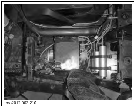
TYPICAL - ACS COMPRESSOR
