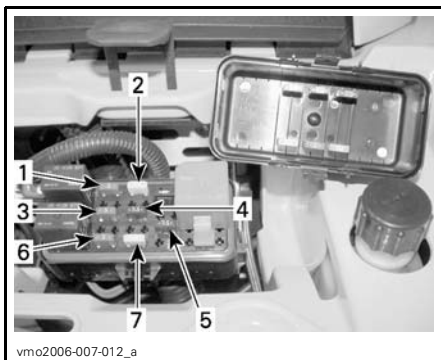
vmr2006-007-012_a TYPICAL — FRONT FUSES LOCATION
