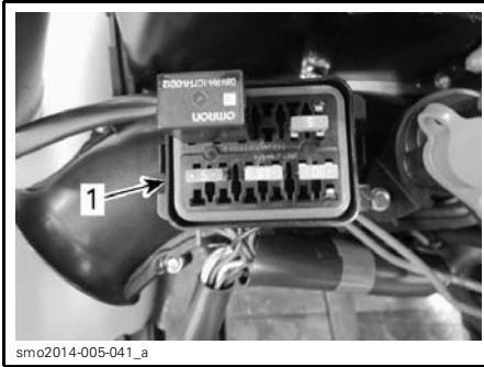
TYPICAL - FUSE BOX COVER REMOVED
