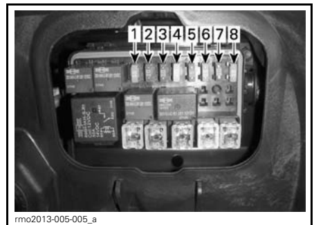
FUSES - LEFT FUSE BOX
