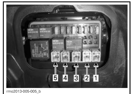
JCASE FUSES - LEFT FUSE BOX
