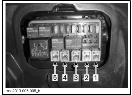
JCASE FUSES - LEFT FUSE BOX
