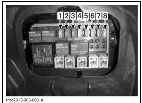
FUSES - LEFT FUSE BOX
